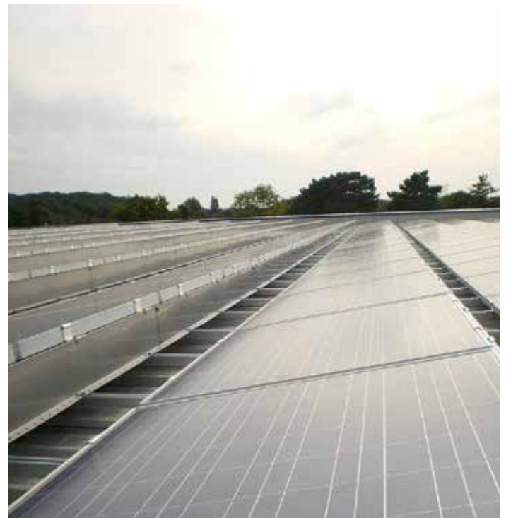
PV mounting system on flat roof, image courtesy of BRE National Solar Centre
