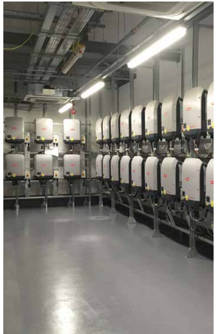
Solar inverter plant room, image courtesy of EvoEnergy
