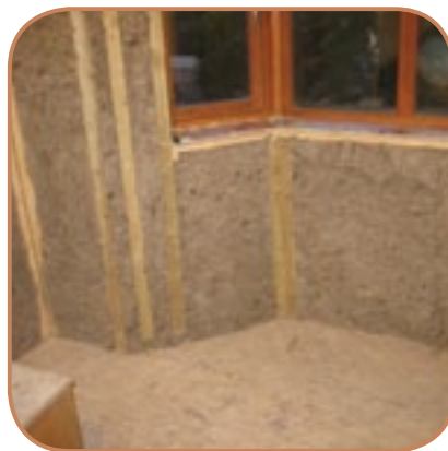
Figure 6.23 Timber stud lining with infill mineral wool or wood fibre insulation. (Source: ECD Architects)
