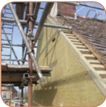
Figure 6.18 Eaves and verge roof structures will need to be extended where EWI thickness exceeds existing overhang dimensions. (Source: ECD Architects)
