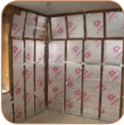
Figure 6.21 Foil-backed polyurethane insulation pinned and foamed to an internal wall. The battens form a service zone ready to receive a plasterboard finish. (Source: ECD Architects)
