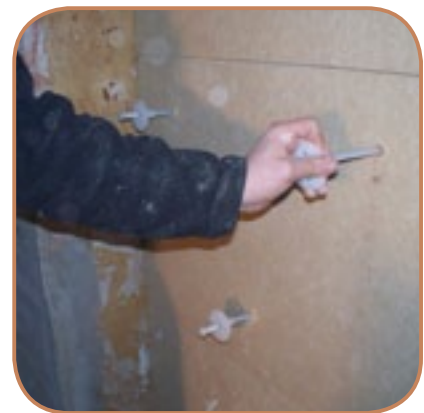
Figure 6.24 Proprietary wood fibre IWI insulation boards being mechanically fixed to an external wall. (Source: ECD Architects)
