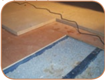
Figure 6.14 Structural support layers and insulation layers can be laid above the joist to eliminate thermal bridges. (Source: ECD Architects)
