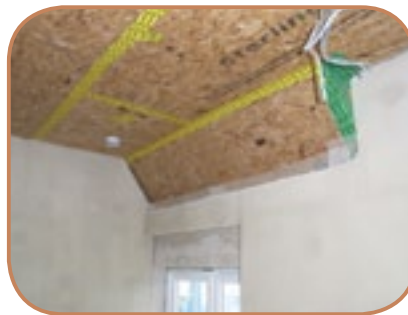
Figure 6.29 Replacement OSB ceiling lining provides an airtight barrier when taped and sealed, as well as providing better support for loft insulation. (Source: ECD Architects)
