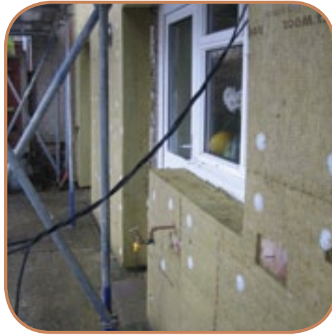
Figure 6.3 External wall insulation has to be restrained mechanically and/or adhesively back to the wall substrate so it must be structurally sound enough to carry the additional load imposed. (Source: ECD Architects)
