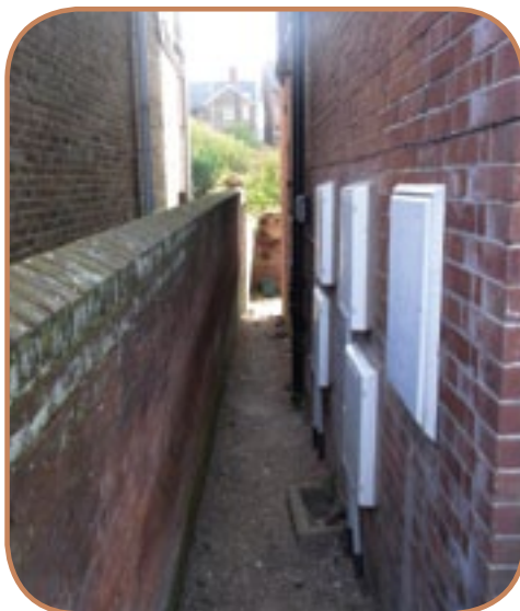
Figure 6.5 Narrow side access with complex external services such as this may restrict options for EWI. (Source: ECD Architects)
