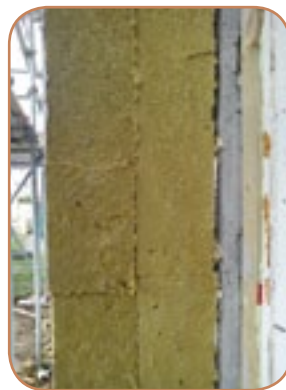
Figure 6.16 Insulated render system build-up: parge coat as air barrier; mechanically and adhesively fixed insulation batts; mesh and base coat render; silicone render top coat. (Source: ECD Architects)
