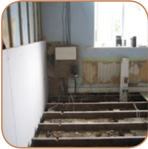
Figure 6.2 Installing internal linings and floor insulation is a very disruptive process and difficult to carry out with residents living in the property. (Source: ECD Architects)
