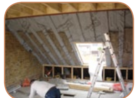
Figure 6.33 An internal roof retrofit showing the breather membrane between and under the retained rafters, ready to receive insulation between and behind them, before the vapour check and dry-lining complete the upgrade. (Source: ECD Architects)
