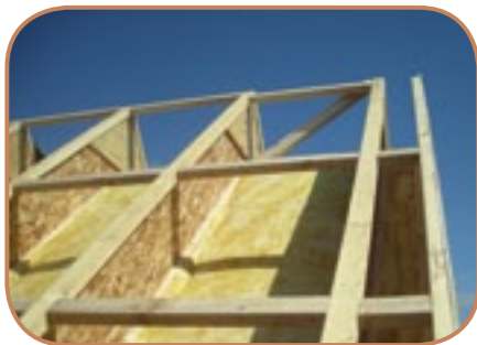
Figure 6.31 I-beam structure over an existing roof ready to receive mineral wool insulation, breather membrane and battens. (Source: Simmonds Mills Architects)
