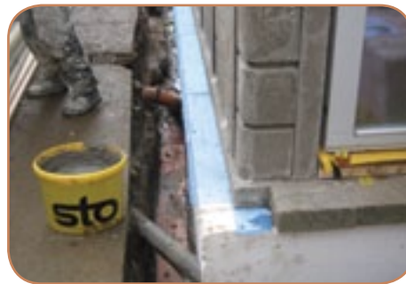
Figure 6.6 Apron insulation extends the heat loss path at the junction of the external walls with the foundations. (Source: ECD Architects)
