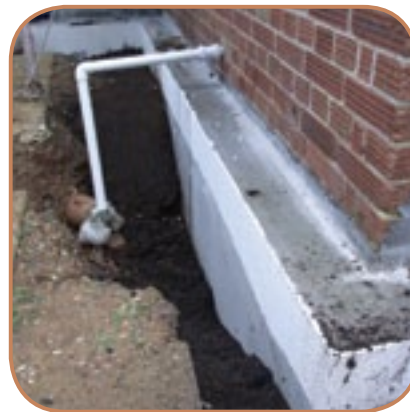
Figure 6.19 Extruded polystyrene insulation installed below ground to insulate floor junctions will require underground drainage systems to be repositioned. (Source: ECD Architects)
