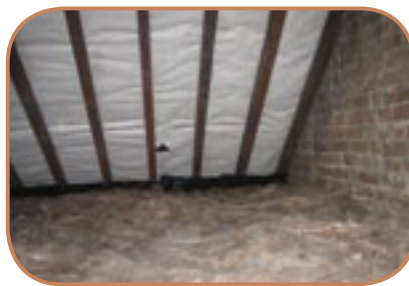
Figure 6.27 Illustration of a cleared, well insulated loft space showing both retrofitted eaves ventilation trays and a vent tile above well fitted mineral wool batts. (Source: ECD Architects)
