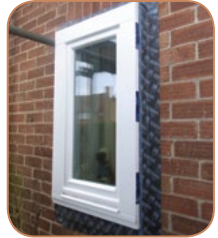
Figure 6.41 Planted high performance window taped to masonry ready for parge coat to be applied and lapped. (Source: ECD Architects)
