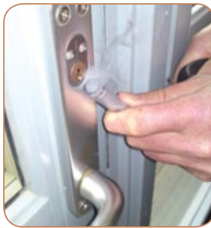
Figure 6.11 Localised testing can be carried out using a smoke pencil to determine the sources of air leakage. (Source: ECD Architects)
