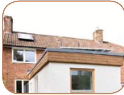
Figure 6.35 Higher performance insulation often means a deeper fascia, which requires aesthetic consideration. In this example, Thermowood cladding has been used. (Source: ECD Architects)
