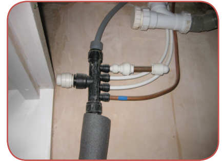
Figure 7.13 Distributing in microbore pipework can reduce dead legs, saving energy and water. (Source: John Willoughby)
