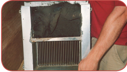
Figure 7.7 Heat recovery ventilation systems need maintenance. (Source: Envirovent)
