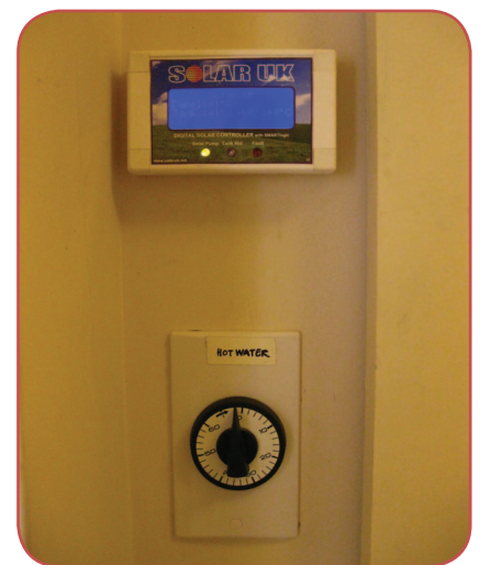
Figure 7.15 A simple runback timer allows the boiler to be used to top up the solar system if the temperatures displayed on the solar controller require it. (Source: John Willoughby)
