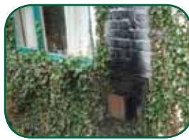
Figure 9.8 A blocked flue? (Source: Carl Harvey of My Home Survey Ltd)
