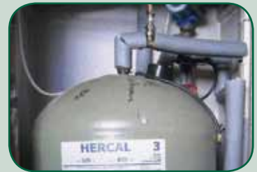
Figure 9.4.1 Hot water cylinder.
