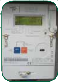
Figure 9.19 A "smart" meter.
